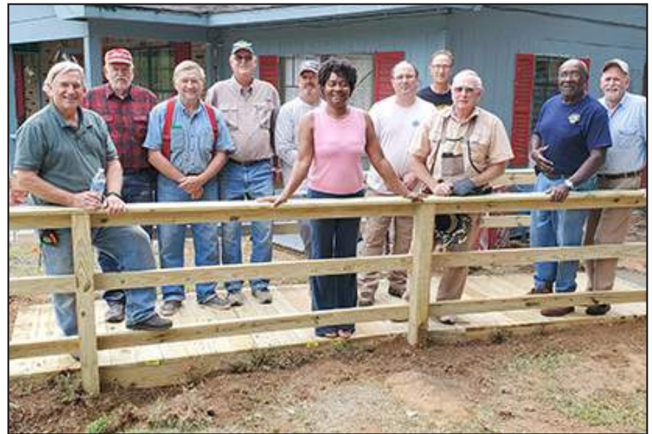
What an awesome day today!!! Bethel Church of Christ of Athens and Alabama Department of Rehab Services joined forces with Lions from Northport, Prattville, Center and Athens to traveled to Carrollton to construct a wheelchair bridge for Mr. and Mrs. Joe Walker. For years Mrs. Walker has struggled to push her husband's wheelchair through rough, muddy terrain just to load him into the car for doctors' appointments. The gratitude expressed by this godly lady made the trip exceedingly rewarding.
